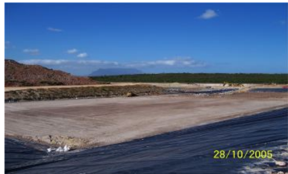
“Monocell” at hazardous waste site
